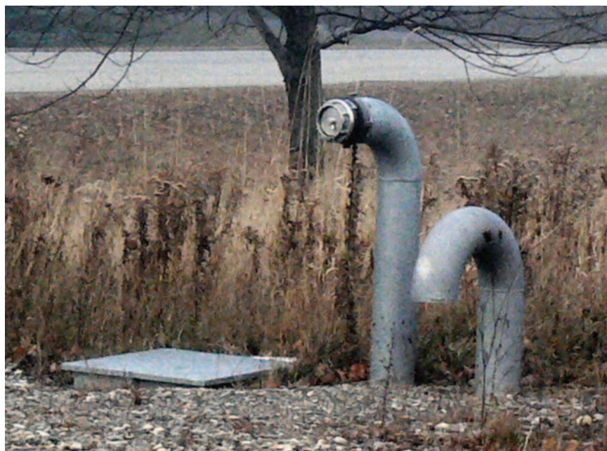
Figure 4.5. Dry hydrant showing all features.
