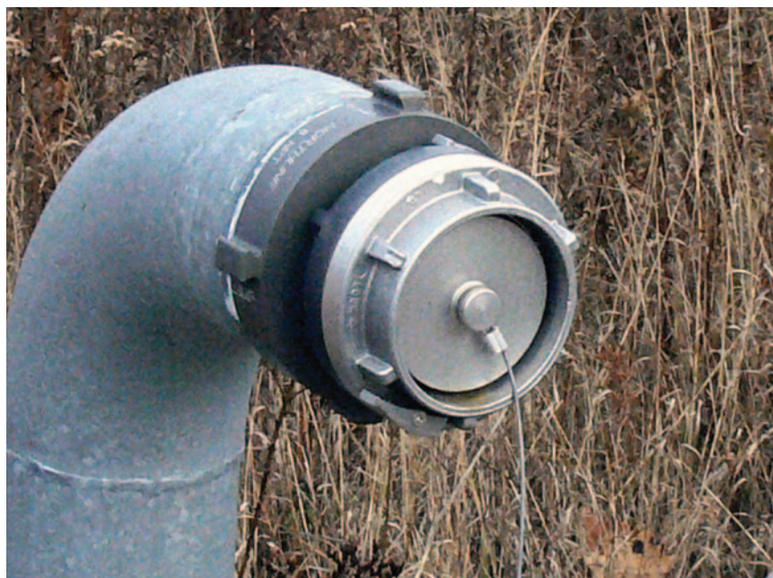
Figure 4.6. Dry hydrant standpipe connection.
