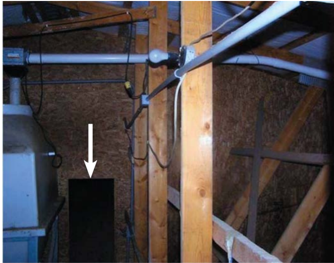
Figure 3.7. This attic fire stop has an opening cut into it (arrow), removing its effectiveness in containing a fire.
