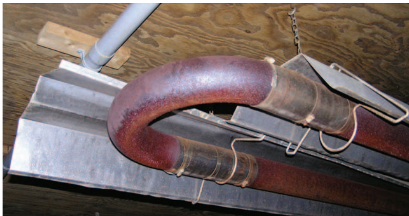
Figure 2.9. Radiant tube heater lacking heat shield. Note close proximity to combustibles (wood ceiling and conduit).
