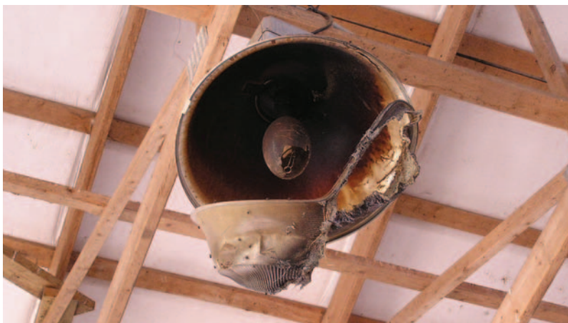
Figure 2.2. Light fixture in a dairy barn that caught fire due to the presence of a bird’s nest (proximity of combustibles). (Photo credit: R. Drysdale, Farm Mutual Reinsurance Plan)
